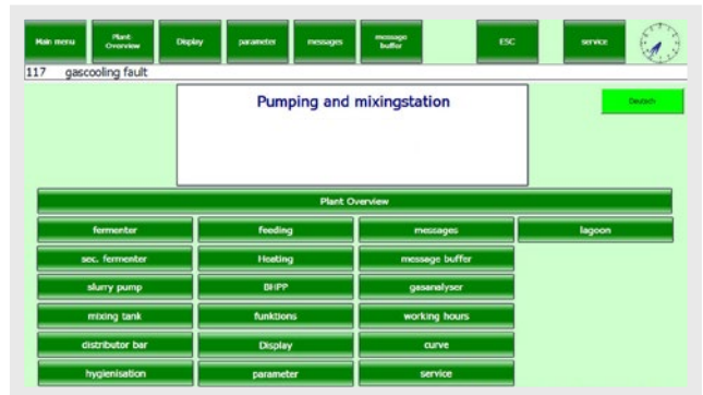
Top-level menu displaying the available submenus, such as Slurry Pump, Mixing Tank, Fermenter, Gasanalyser, Feeding, etc.
