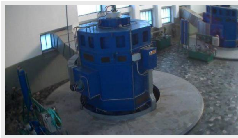
Figure 26. Exposed web camera showing a hydro facility
